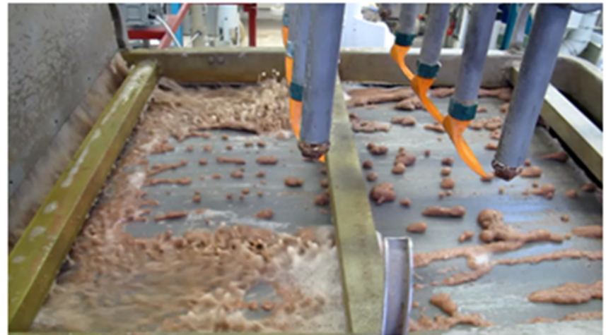
Dewatering, RHEWUM WAFL screen
